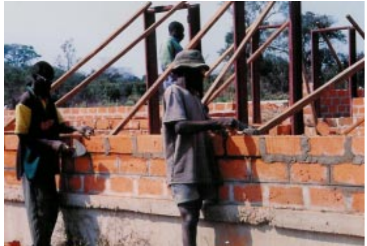
The entire hospital structure was built locally by hand, including the manufacturing of bricks.
